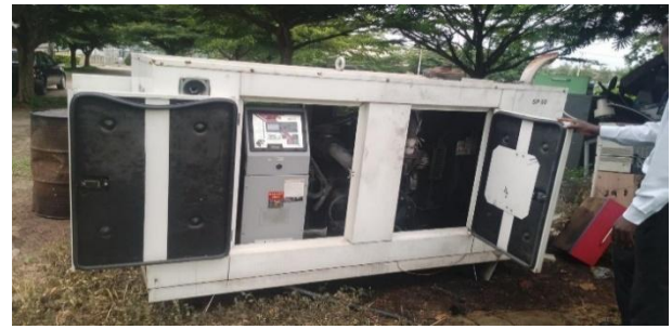
Fig. 5. Mikano SP 60 generator installed at the healthcare facility
