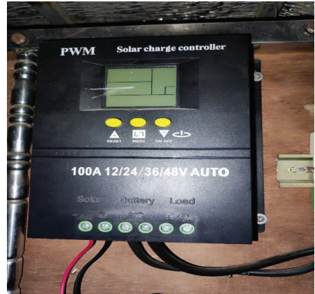
Fig. 3. The solar charge controller
